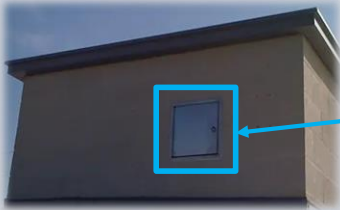
Fire rated access enclosure installed in an elevator hoistway overrun
